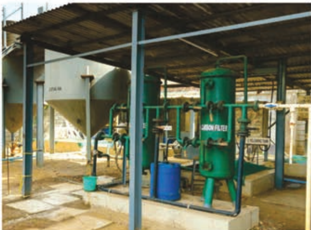
ETP Plant at Unit 1 Vasai
