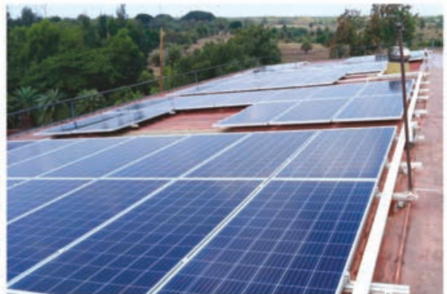
Rooftop Solar Panels at Unit 2 Palghar
